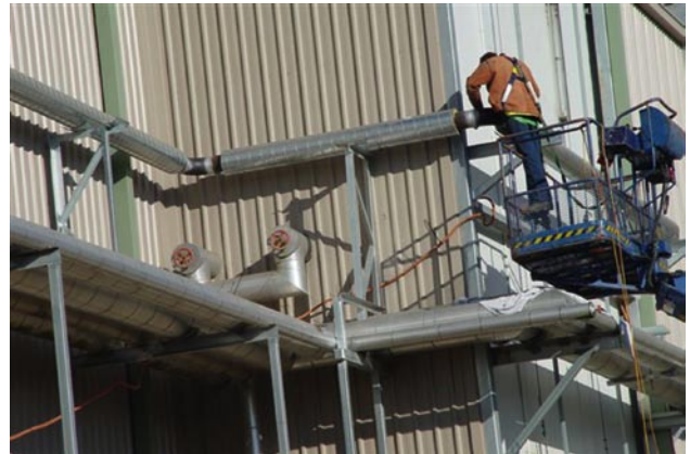
Insulated ammonia lines
