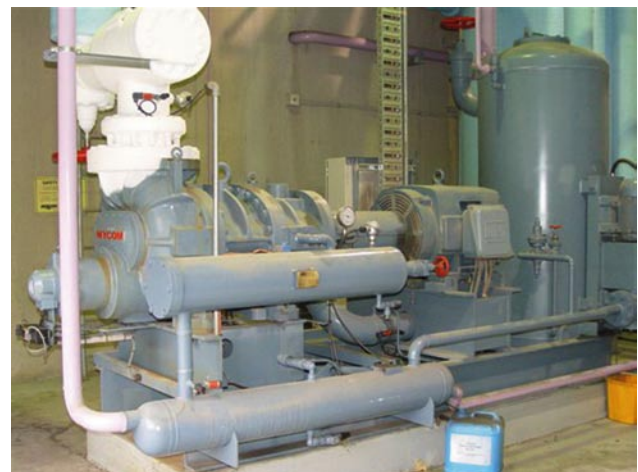
High stage screw compressor
