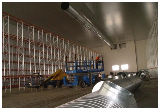
Air distribution ducts
